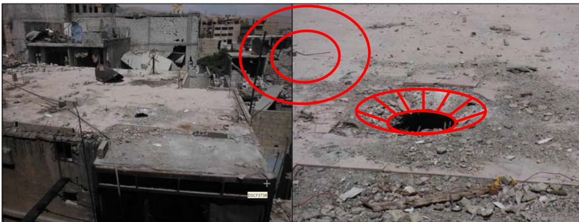
FIGURE A.6.3 ADJACENT ROOF SHOWING A CRATER SIMILAR TO THE ONE ON THE ROOF TERRACE AT LOCATION 2
